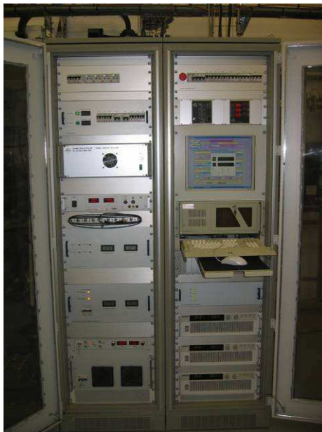
Electronic and Local Command Cabinet
