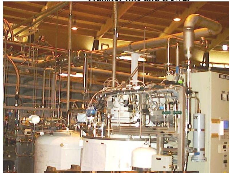
Transfer line and Dewar
