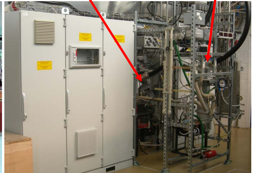
1.3 GHz 30 kW transmitter at the HoBiCaT
