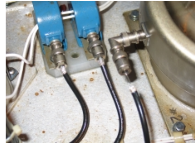
Current and HV probe coaxial cables
