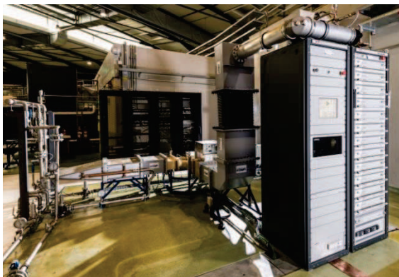
Figure 5: SSPA transmitter for the ALBA booster.
